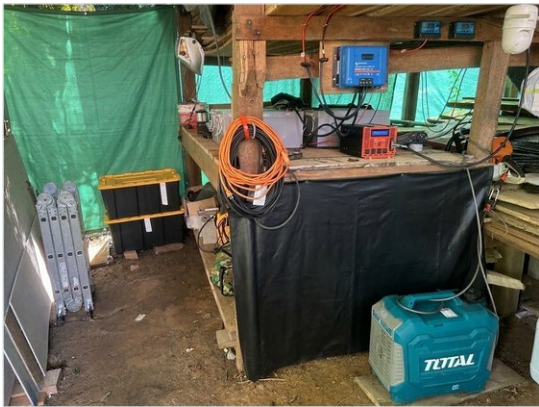
The power station under cover: Victron SmartSolar MPPT and auxiliary controllers, inverters, the 900 Ah battery bank and the backup generator.
